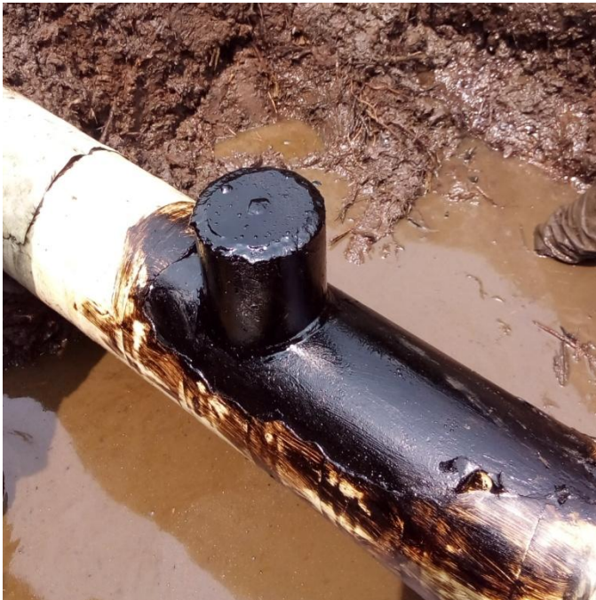
Fig C: Spill point covered with a cone
