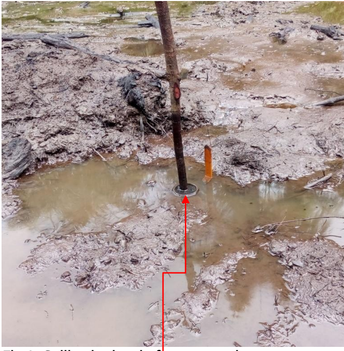
Fig A: Spill point just before excavation
