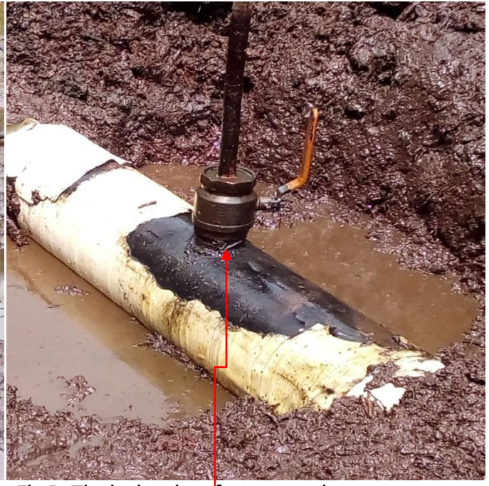
Fig B: The leak point after excavation
